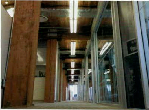
The interior of 564 Beatty: rather than gut the old building, floors, columns, ceilings and walls were maintained and reinforced to modern seismic standards | GLEN STOKES
